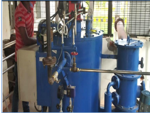
Figure 2:- Process Boiler used in dairy industry
